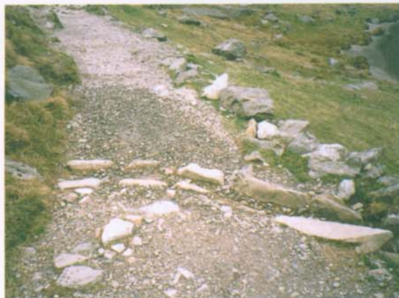
Poor design of drain - inadequate size and requiring continual maintenance
