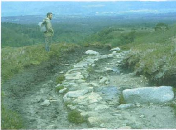
Failed built path - poor design compounded by lack of maintenance
