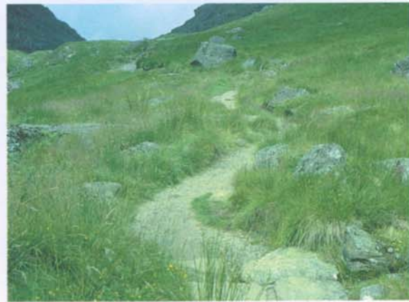
After - erosion stalled with pre-emptive path definition and landscaping
