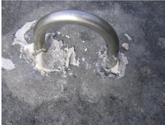
Staple, showing R leg failure
